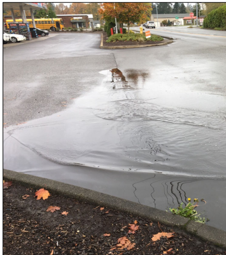
Ponding at QFC parking lot entrance.
