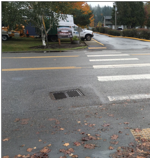
Poorly placed surface inlet in curb lane.
