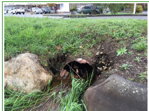
Stormwater Infrastructure Challenges
