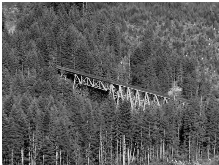
This historic steel bridge over Vance Creek once supported a logging railroad and may be well suited to conversion to a multi-use trail. The area is owned by Green Diamond Resource Company.
