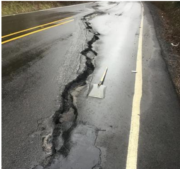
Figure 8-12 Highway 302 Landslide East of Victor (2022)
