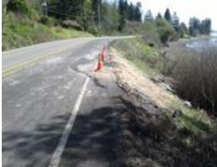
Figure 8-11 SR 302 Slope Erosion Near Victor
