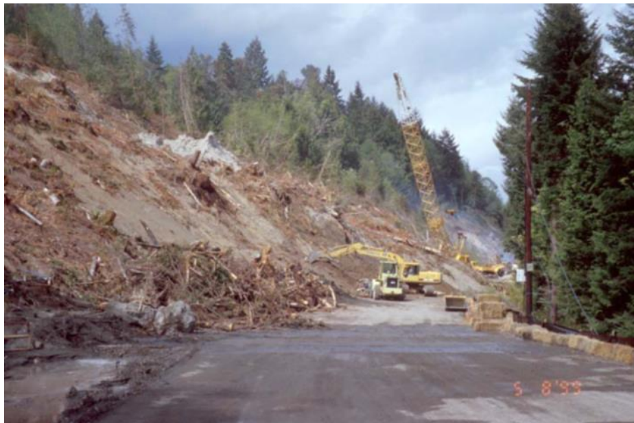
Figure 8-8 Highway Closure at Jorstad Landslide – Winter 1998-1999
